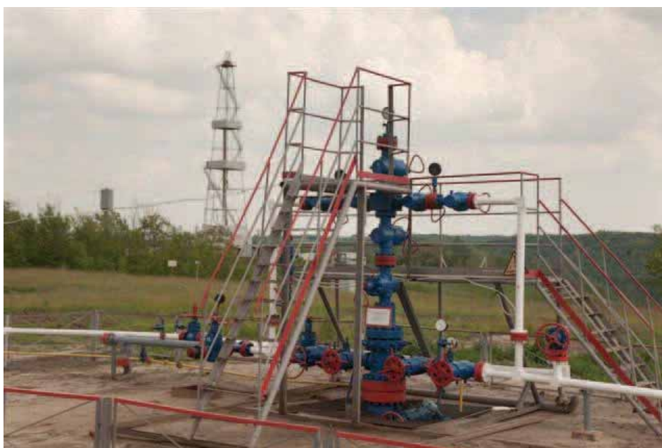
Figure 6: Wellhead assembly, Lutsenkivske field, well 13
