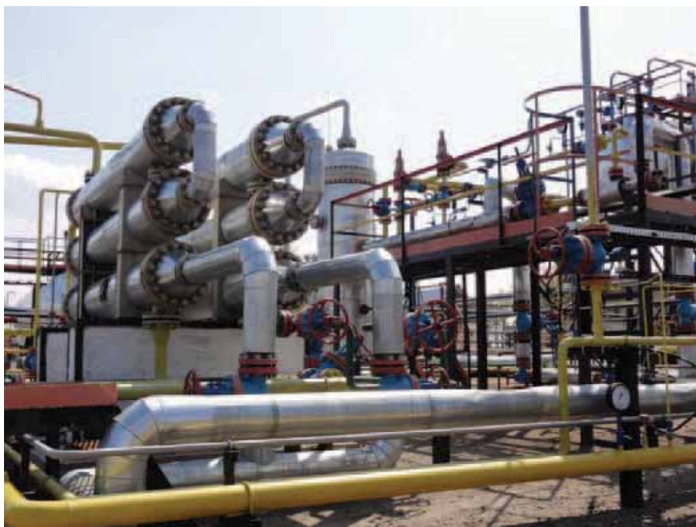
Figure 3: Gas Plant processing production from Berestivske field
