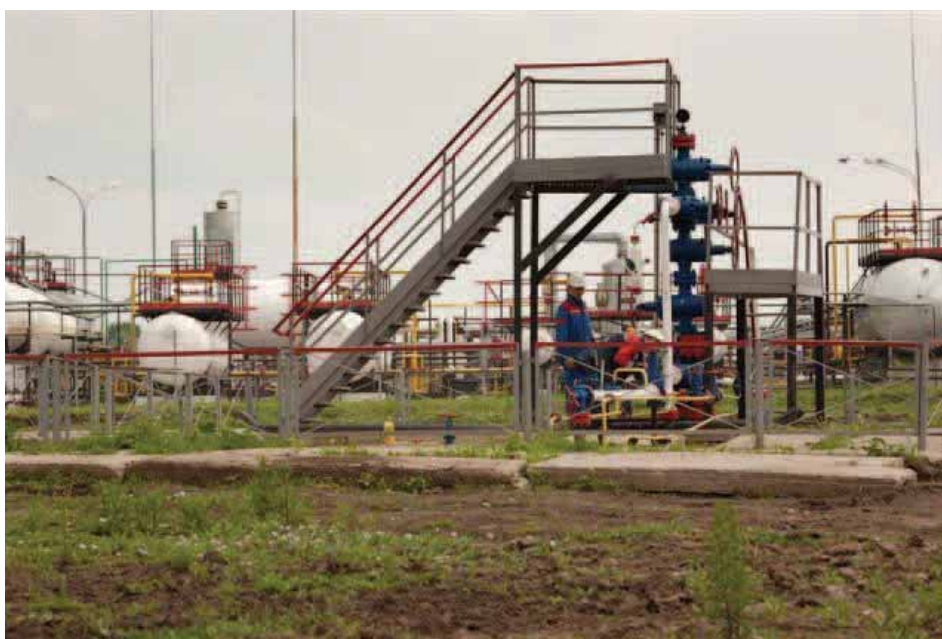
Figure 8: Processing tanks and wellhead assembly, Lutsenkivske field, Well 9
